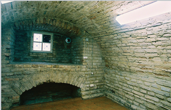
Cellars. In one such cellar, monastery beer was brewed. It seems that the low opening cut out in the niche was used to release water into the Kačerga Brook. In the cellar there are stairs leading down from the courtyard. There used to be a well in the nearby courtyard. Photo by A. Pliadis.
