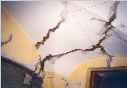
Cracks in the vaults and walls uncovered during the last renovation. The building may have been damaged following the reconstruction at the end of the 19 th century when the height of the building was increased. Photo by E. Purlys.
